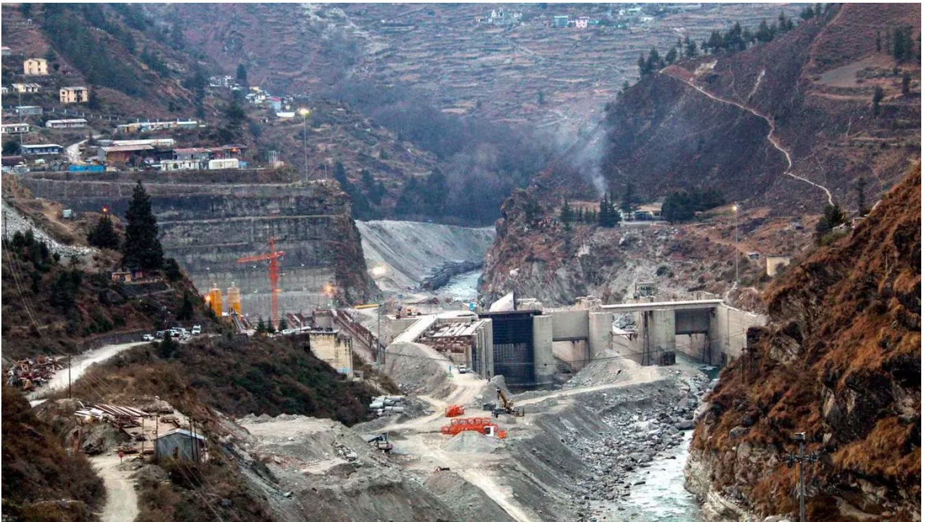
Image 3: Tapovan Vishnugad Hydropower Plant of NTPC, in Joshimath, Tuesday, Jan. 17, 2023. Source: PTI
